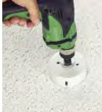
1 Cut hole in the desired location in the ceiling with 4" hole saw.
